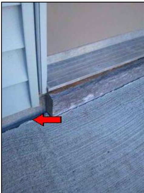
Concrete separated from foundation rear patio
