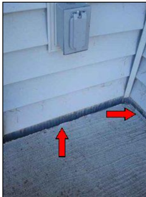
Concrete separated from foundation rear patio
