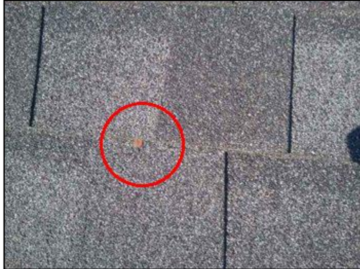
exposed fastener / granule loss
